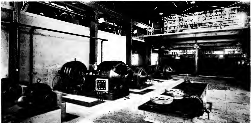
Interior of the power house at the sending station Bolinas, California, showing 300 k. w. motor generator sets and control board.
